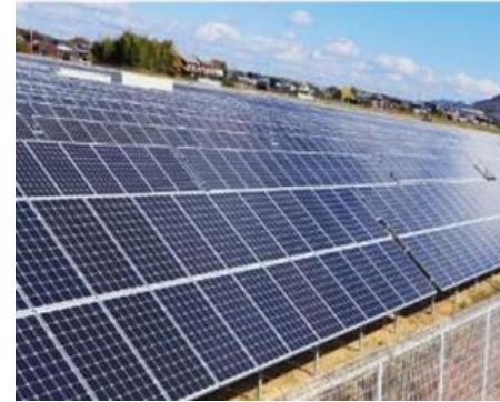
Kobe Bussan's Solar Power Plant
