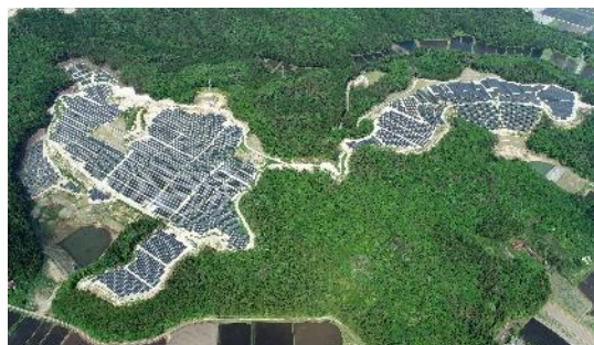
Kobe Bussan's Solar Power Plant (Photo: Nishishirakawa Power Plant with the capacity of 18.9 MW, which started operations in June 2022)
